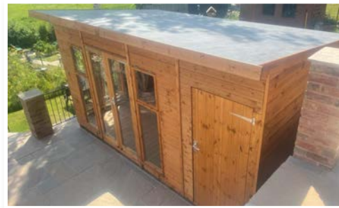
EPDM rubber roof
